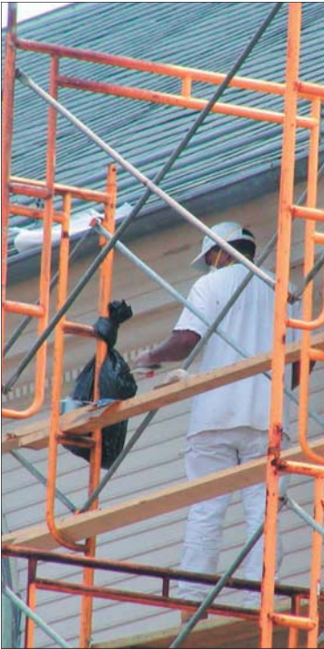
Great care should be taken when removing old paint, especially if you suspect that there is lead in it. This man, working high above the ground on Trinity Church, is taking proper precautions while removing old paint by wearing a face mask and gloves. Using a hand-scraping technique is the best way to remove paint to minimize the chance of damaging historic
